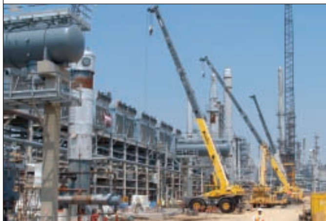
Construction is underway on the new processing units that will produce cleaner diesel fuel to meet new federal requirements starting in June 2006. The new units are scheduled to be completed next spring.
